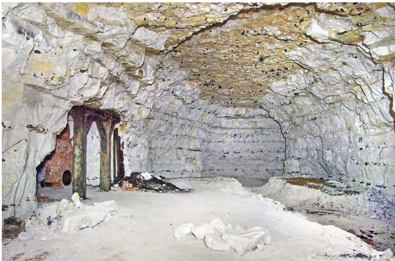
Chalk mine main roadway outside the Council repository, the brick outer wall of which can be seen to be set back from the main mine wall
